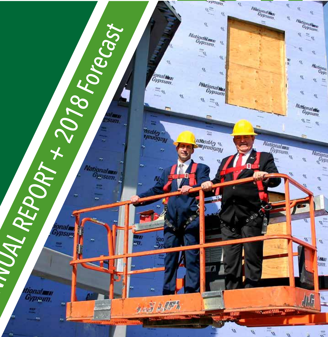
Heath Talhelm, Town Council President and Walter Bietsch, Mayor at the Utility Departments' addition under construction.
