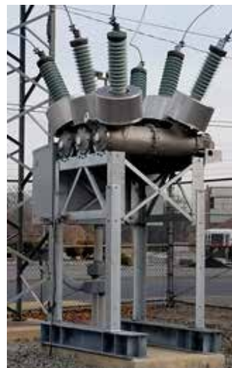
New Grant Street Substation Circuit Breaker
